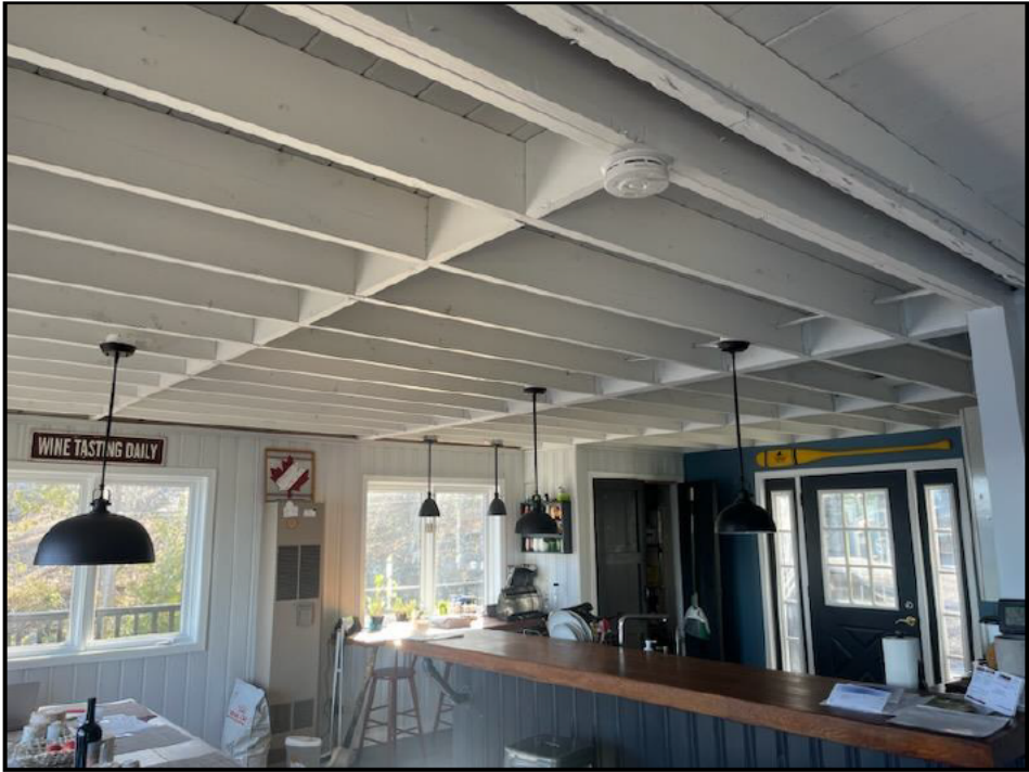
Photo 4 – Over spanned 2 nd Floor Framing
