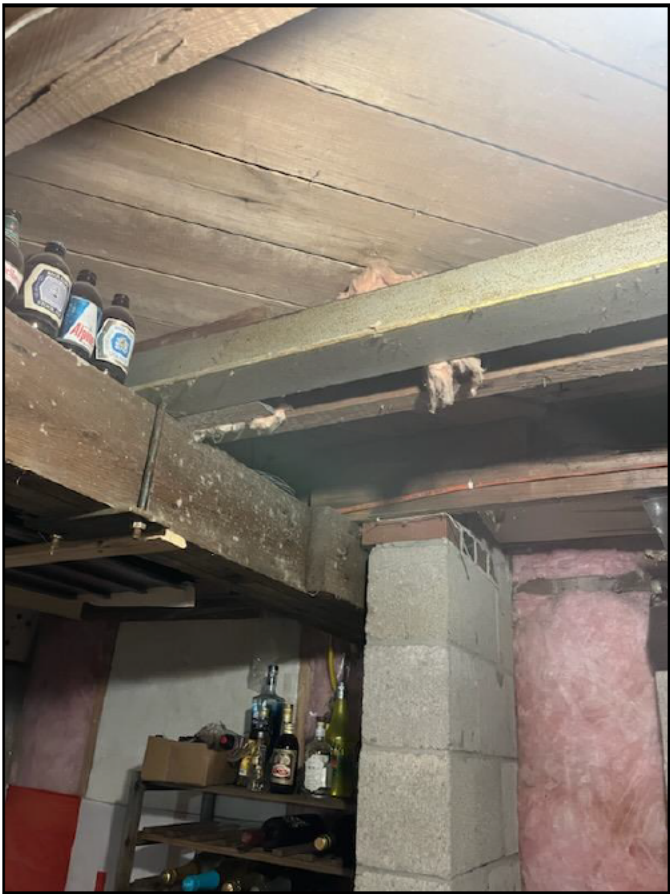
Photo 5 – Lack of Building Envelope
